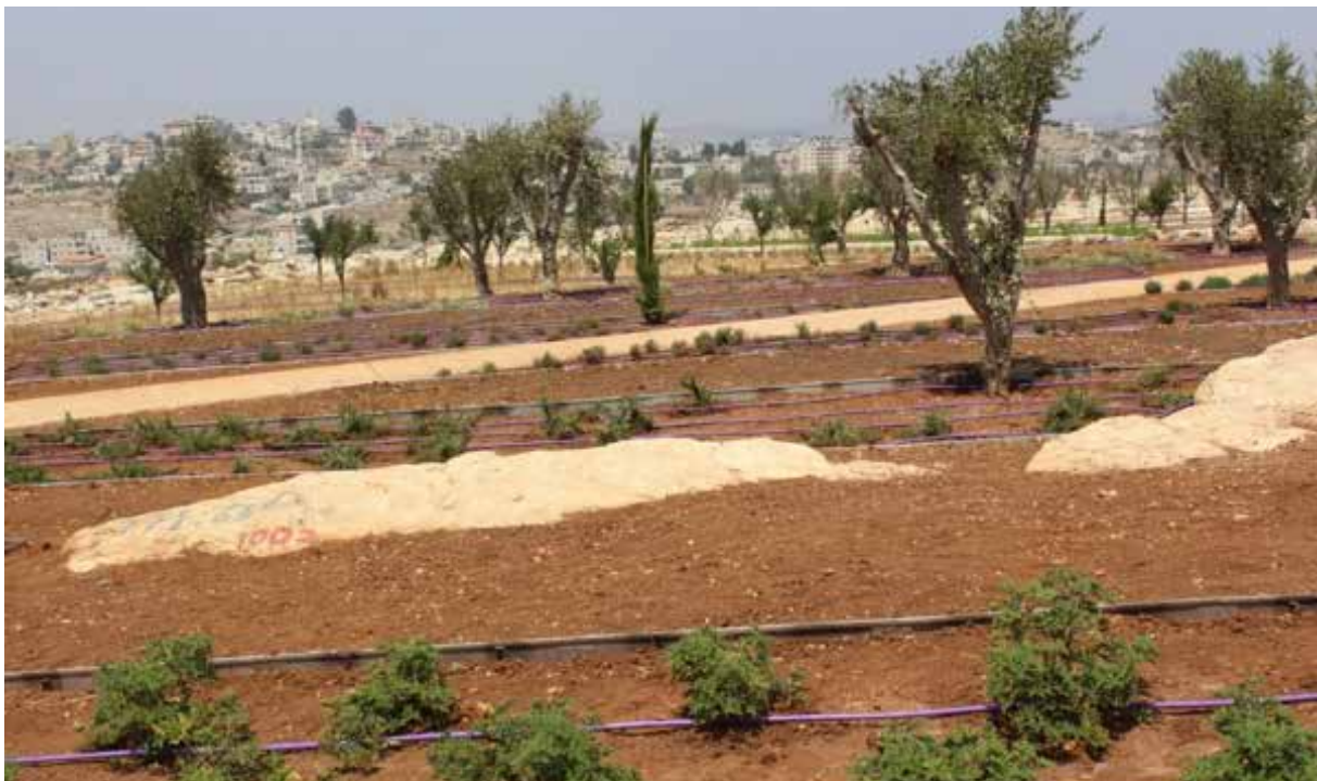
Figure 11: Drip irrigation system for landscaping
