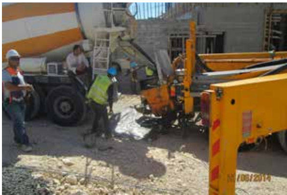
Figure 19: Concrete waste management
