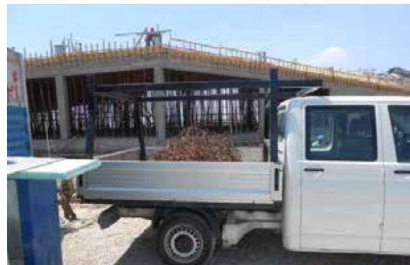
Figure 17: Collection of recyclable scrap steel & transferring it to construction waste management area
